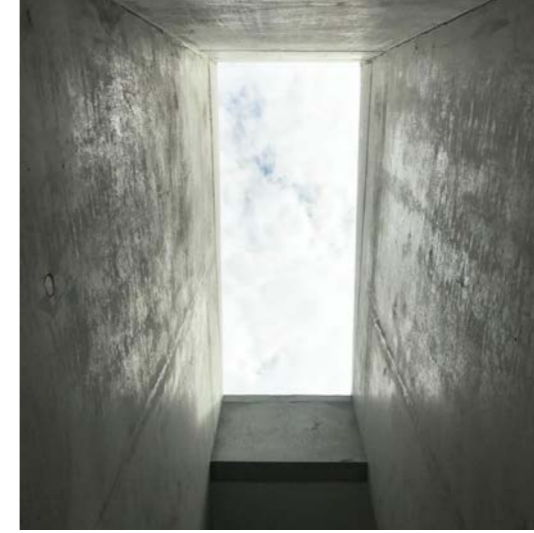
Overlys i trapp, skjult ramme
