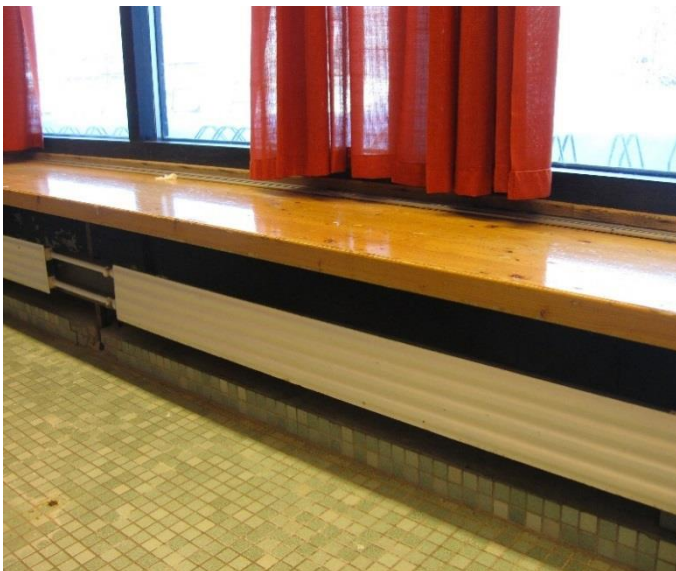
Vegg under vindusfelt
