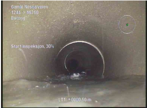
13.11.2024 144510_15750_1244_13112024_024601_037.jpg, 00:00:00, 0.50m Start inspeksjon, 30% / Rennende vann
