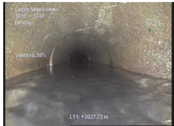
14.11.2024 150201_1016_1049_14112024_030307_043.jpg, 00:02:40, 27.70m Vannivå, 50%
