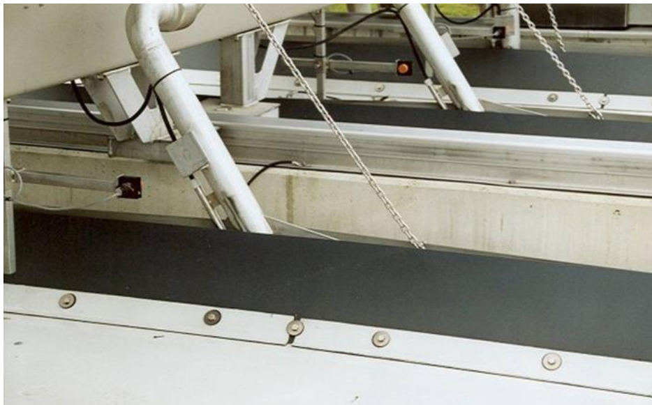
Fig 11: Odor covers with shaft passing through a flexible rubber material
