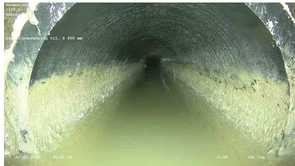
22641_3355_70162_Veumveien_020221_102428_014.jpg, 00:14:45, 196.20m Dimensjonsendring til, S 450 mm / Mindre dim
