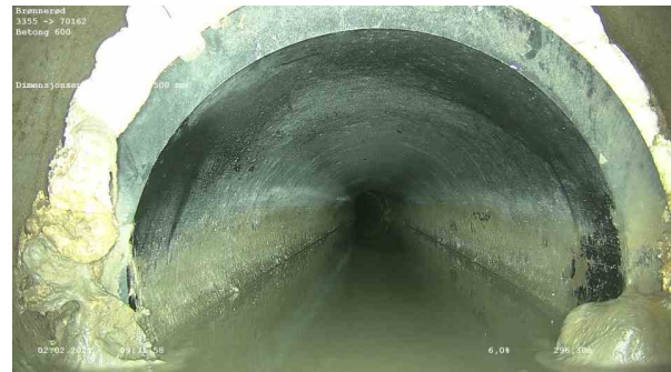
22641_3355_70162_Brønnerød_020221_090048_007.jpg, 00:26:02, 296.30m Dimensjonsendring til, S 500 mm
