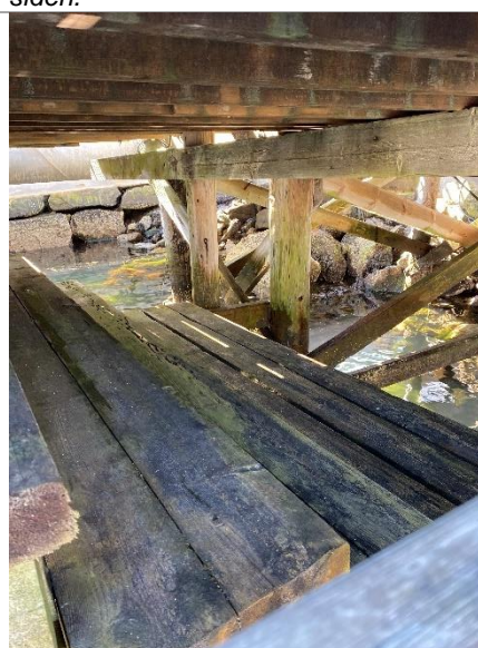
Bilde 19: Trapp under kai/aggregatthuss.
