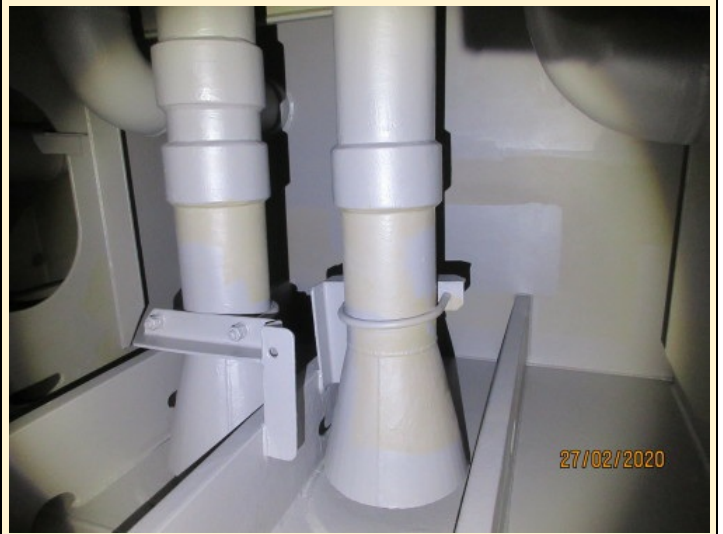
40P WB T/U Inspection.
