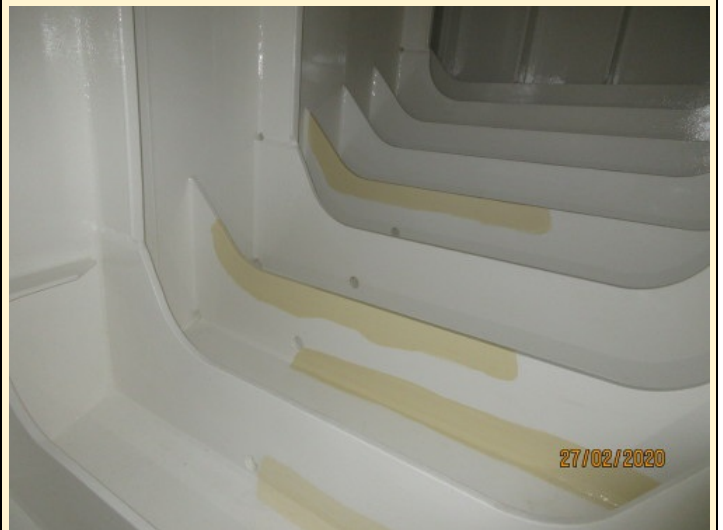
162P FW T/U Inspection. 2xcream color, lack of white.
