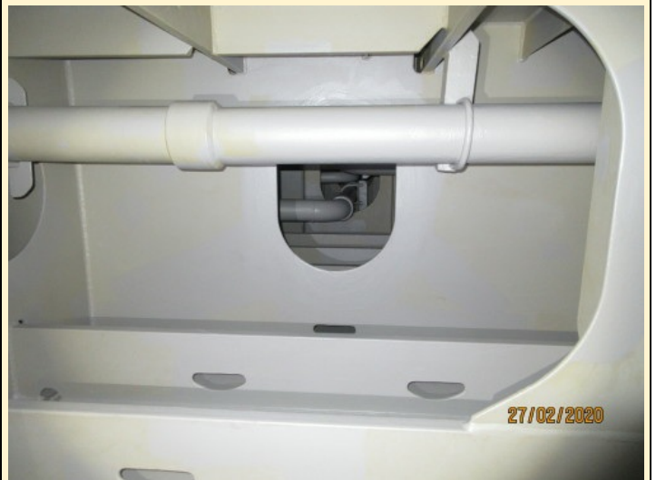
40P WB T/U Inspection.
