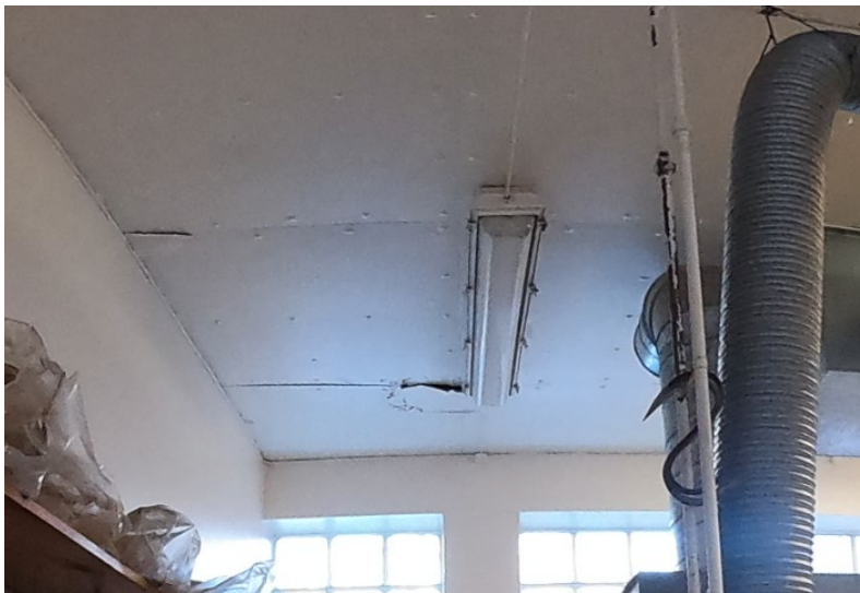
B4.1 – Asbestplater i taket, PCB lampe
