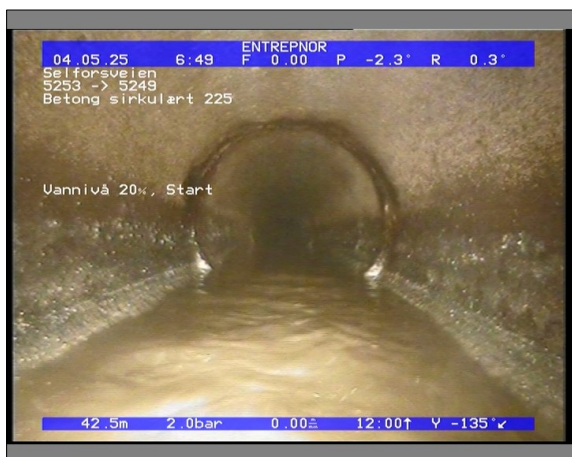
Foto: 5854_5249_5253_05022021_044248.JPG 42,58m, Vannivå 20%, Start
