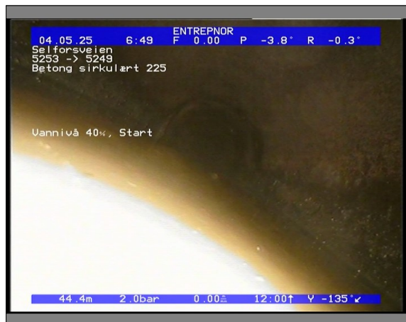
Foto: 5854_5249_5253_05022021_044331.JPG 44,41m, Vannivå 40%, Start
