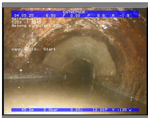
Foto: 5854_5249_5253_05022021_044413.JPG 45,28m, Vannivå 10%, Start
