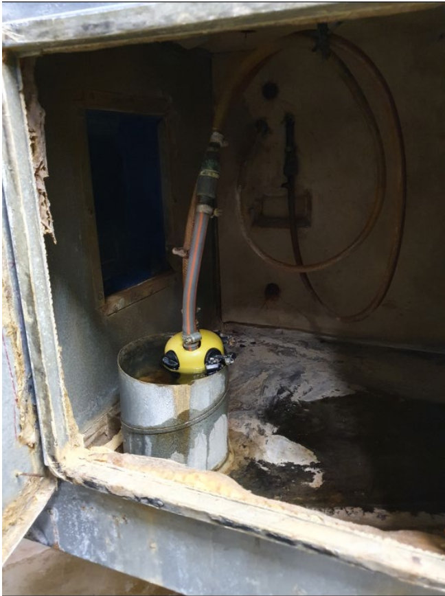
Picture 6. Inside the air treatment cabinet where the old system must be replaced for the new system
