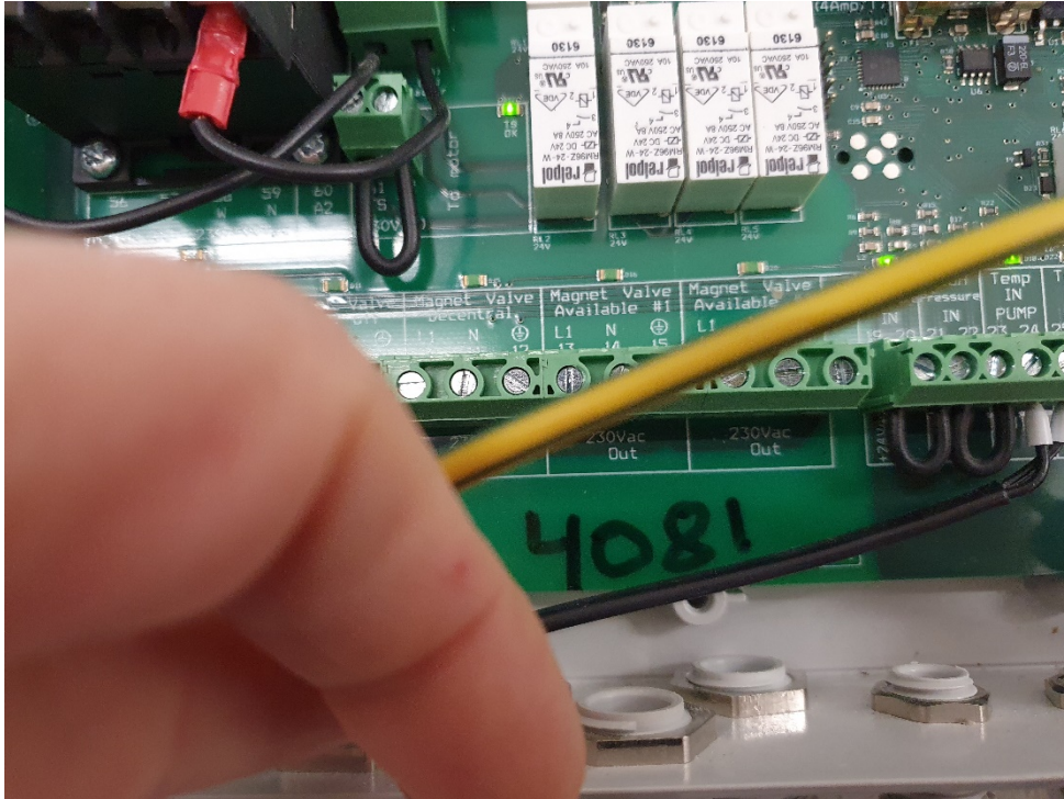
Picture 2. Pro Air number of the installation
