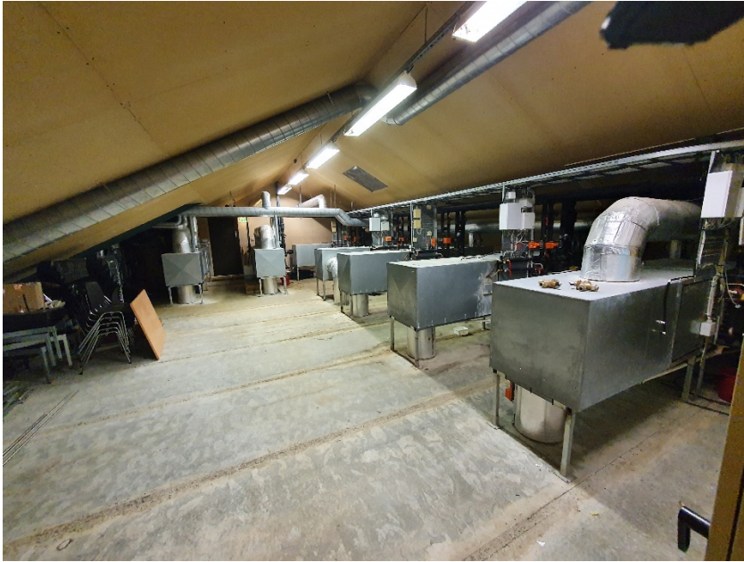
Picture 4: rom on the second floor, where the air treatment cabinets have been placed
