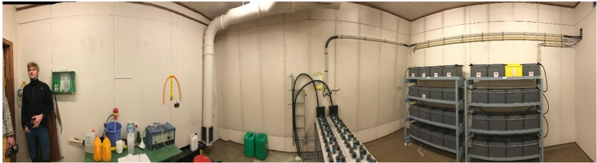
Figure 4 Panorama picture of the Battery Room
