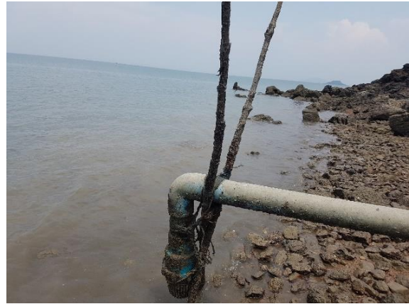
The water intake should be moved further out from the shoreline
