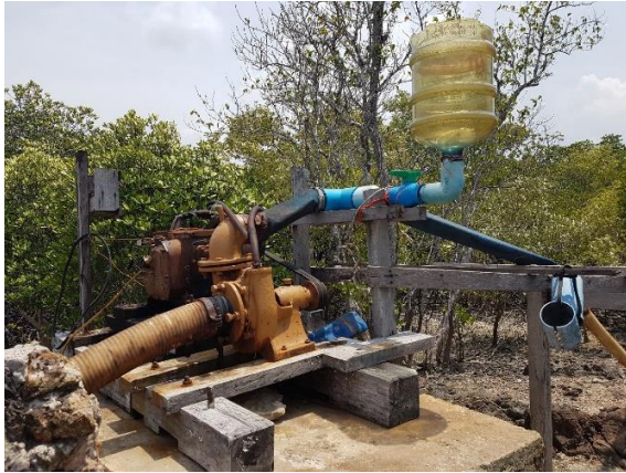
The seawater pump needs to be replaced
