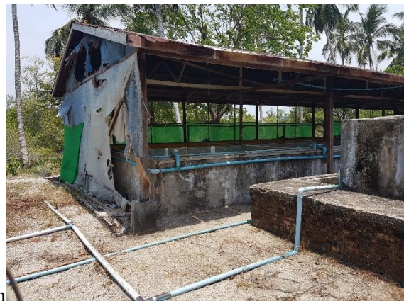
Some of the buildings need to be repaired
