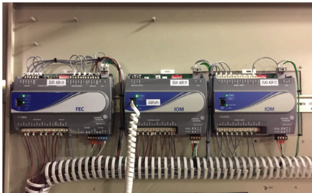
Figur 5.6.0-0: Johnson Controls Field Equipment Controller (FEC) / Input / Output Moduls (IOM).
